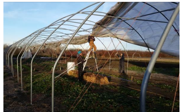
Fig. 10. Supersolo tunnel with cover parked half way up the side of the tunnel in fall of 2015.
